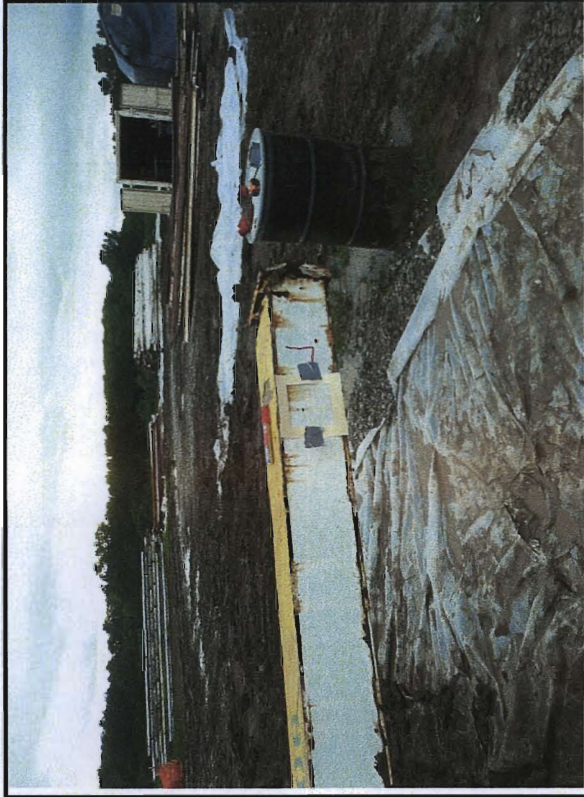
Photograph 56 | Wipe Sample Location # 719L3
